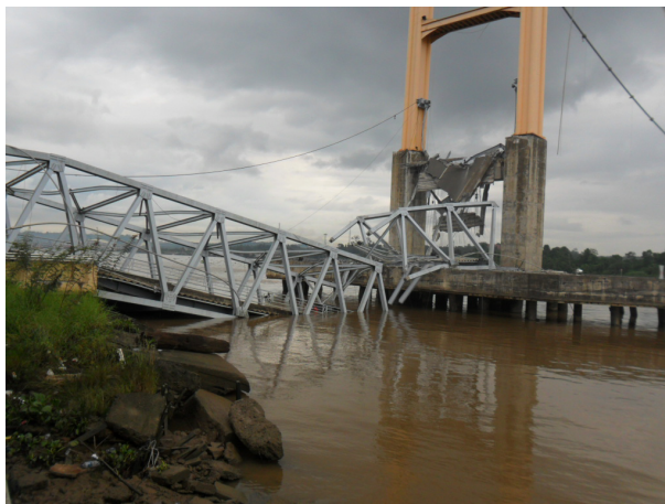
FIGURE 1. The collapsed Kutai Kertanegara bridge [1]
